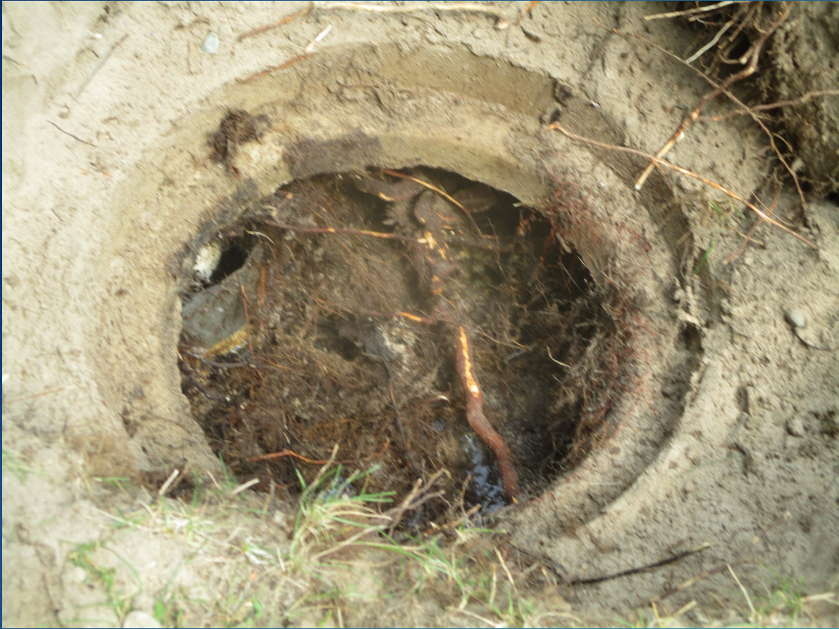
← Roots in the tank
