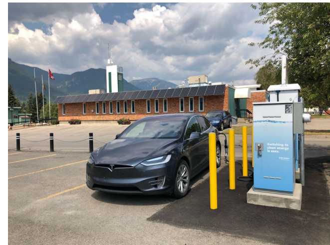
Level 3 DC Fast Charging station in a small BC community as part of Accelerate Kootenays
