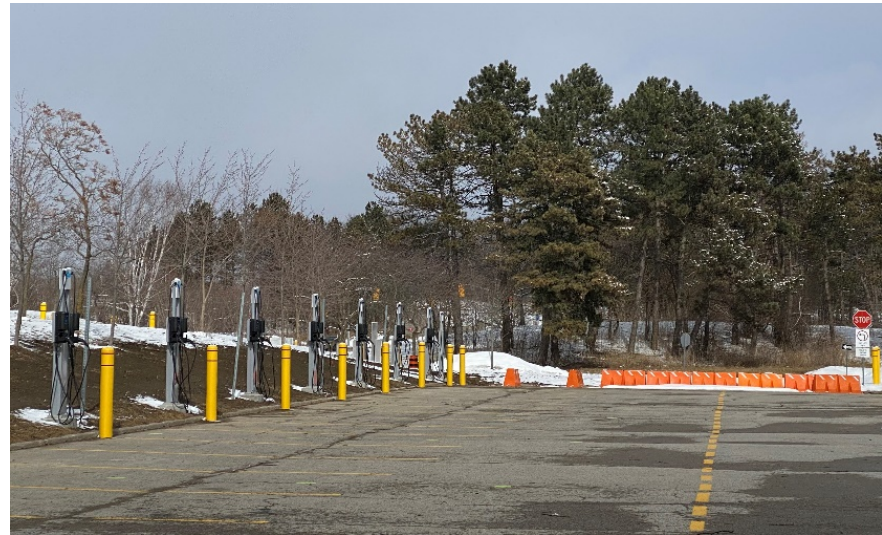
Bank of Level 2 charging stations installed in Toronto Zoo carpark.
