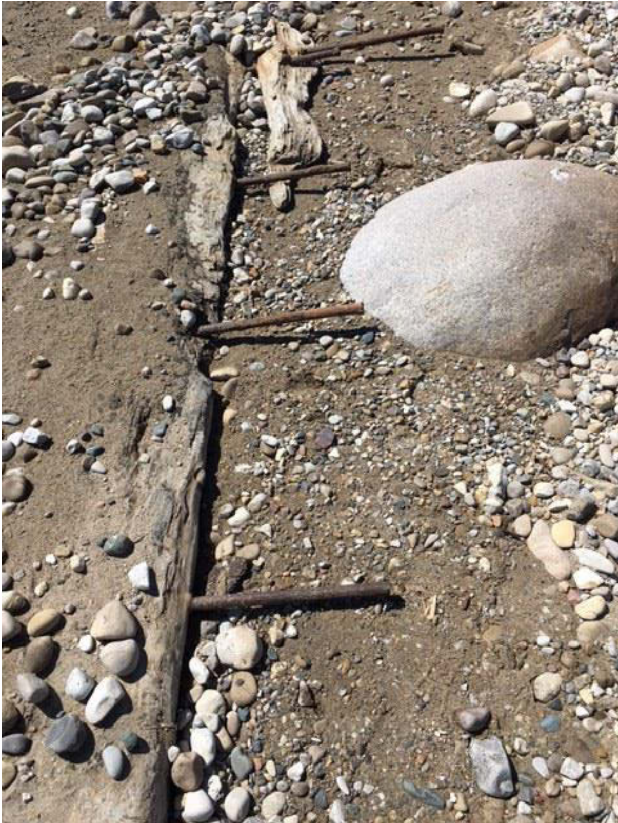
Photograph 5: Extension of Iron Through Bolts Suggesting Another Plank (May 2021)
