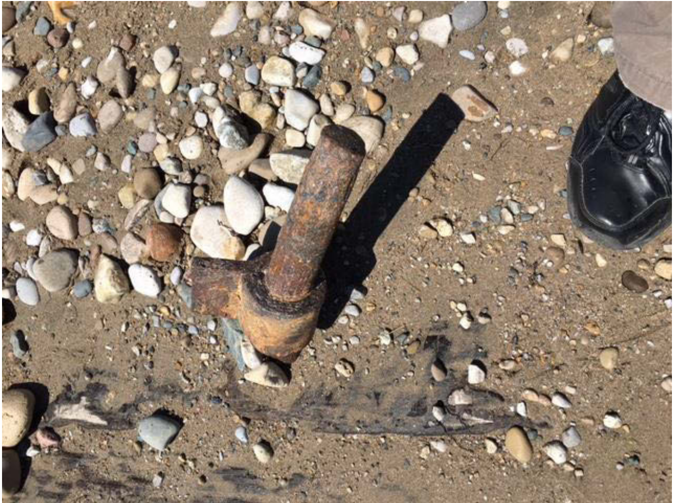
Photograph 11: Pivot Pin Coming Through Planking (May 2021)
